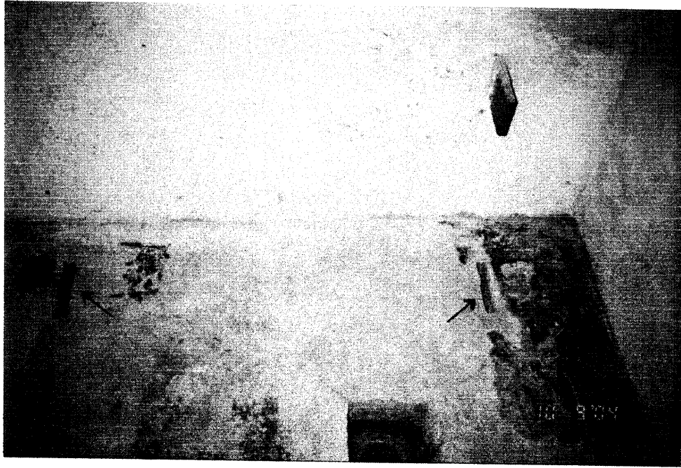
Figure 21 - The arrows point to two holes in the concrete floor which held the shelf support boards. This photo also shows the position relationship of the floor holes, the square hole in floor, and the only remaining wood shelf support in wall.
