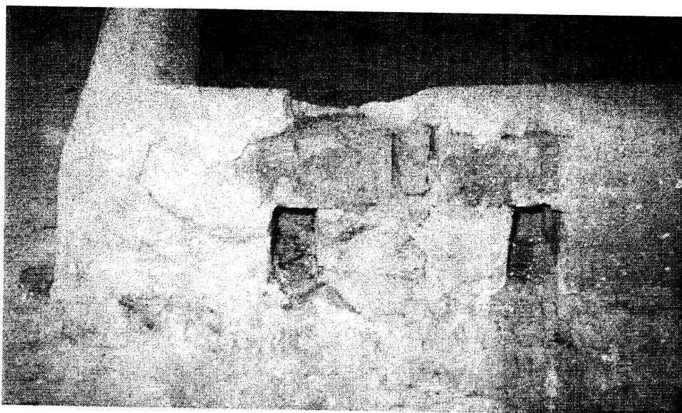
Figure 18 - Two of the five drain holes in the processing pan are shown. These holes were formed around red bricks seen in here where the cement has broken off.
