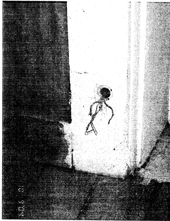
Figure 25 - Room E-1 in Assay Building. Telephone wires in door casing.
